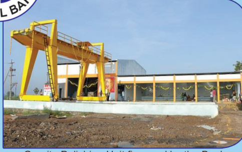
Granite Polishing Unit financed by the Bank
